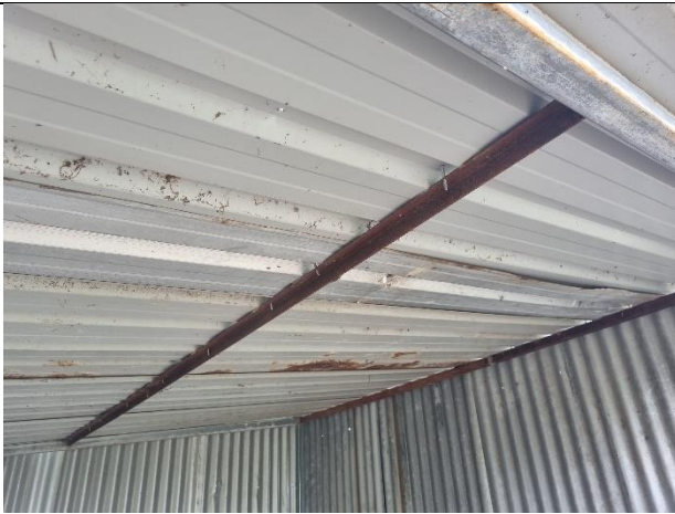
Photo 15: Animal shelters 5 and 6 equal angle purlins – to be replaced
