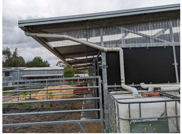
Photo 22: Southern roof drainage repaired
