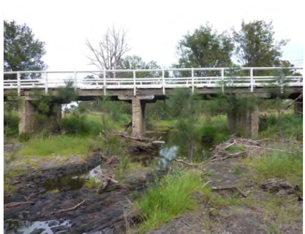
Timber Bridge due for replacement
