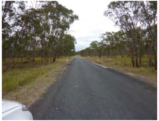
Sealed Road – Condition 2 (Torryburn Road)
