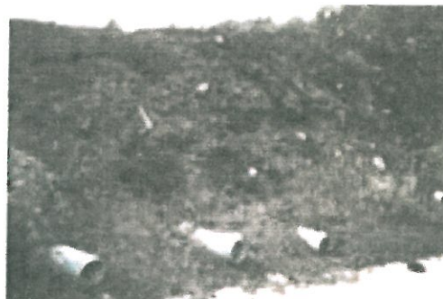
Example of a passively aerated windrow with aeration pipes visible
